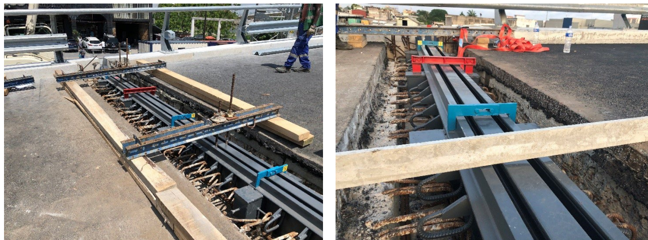
→ Expansion joint being adjusted to the definitive position. Aluminium bar checking alignment with the road.
